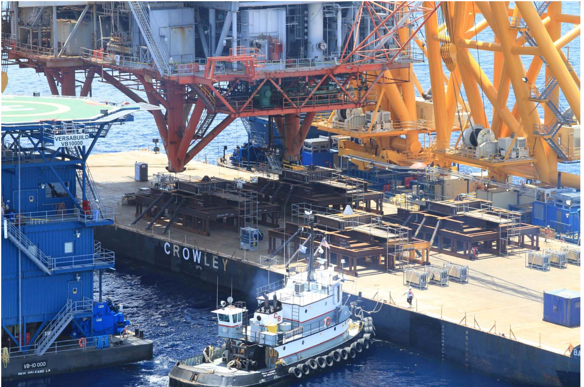
Using tugs and tugger winches, the barge is positioned to receive the topside.
