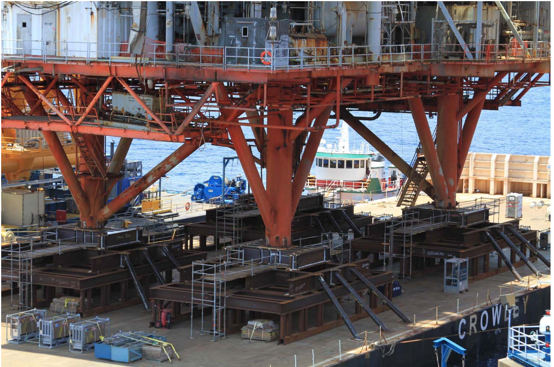
12:50 PM. The VB – 10000 lowers the topside onto the stabbing cones, and releases most of the load.
