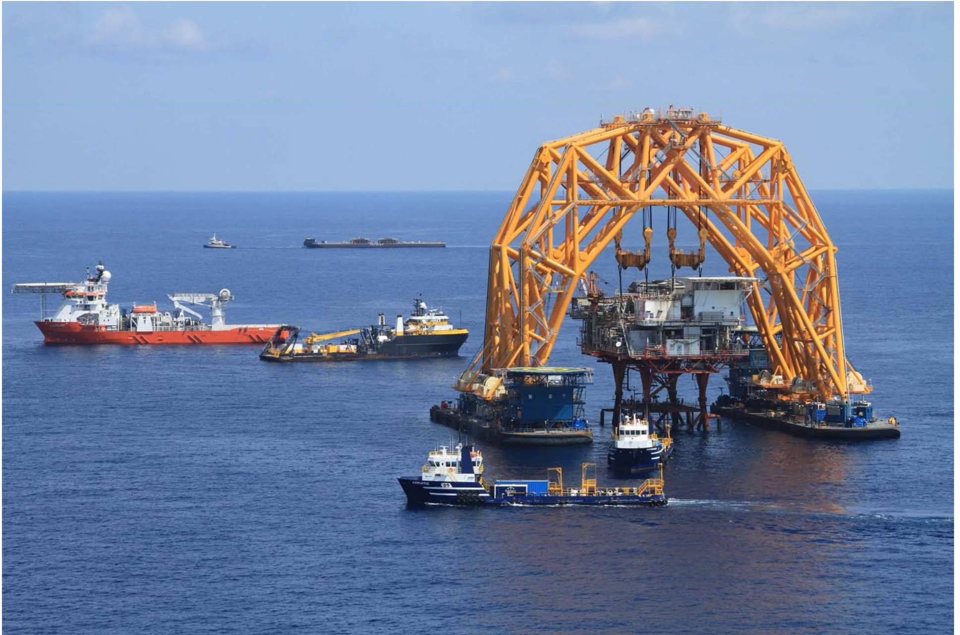
While the cuts are being completed, the transport barge (in the background) is towed into position nearby.
