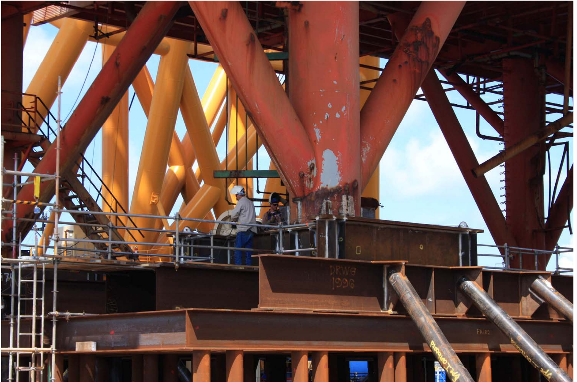
Welders immediately board the barge and begin the work of sea-fastening the topside.
