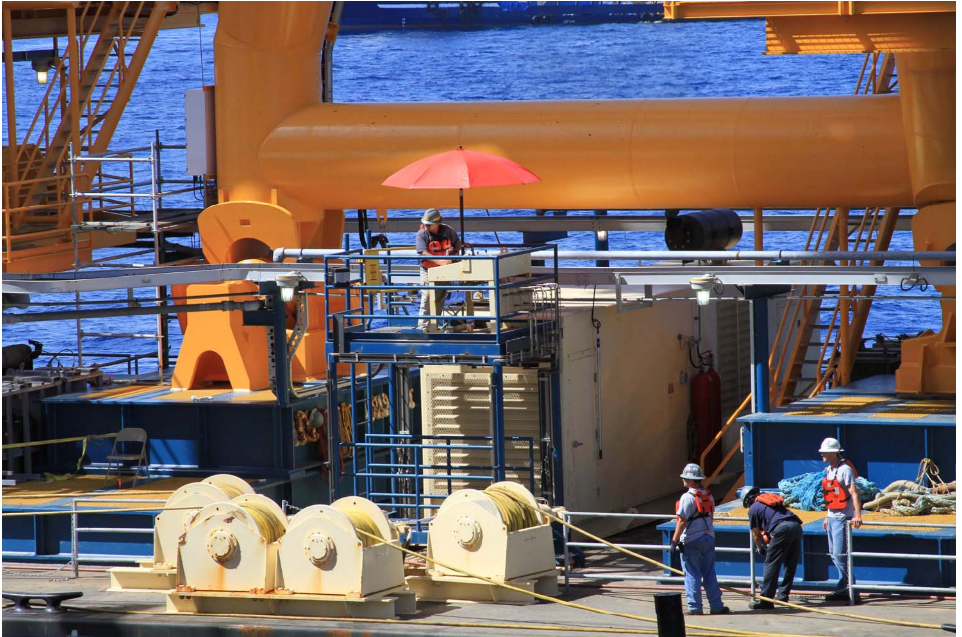
Again the VB – 10000 crew man the tugger winches to guide the transport barge out of its berth.
