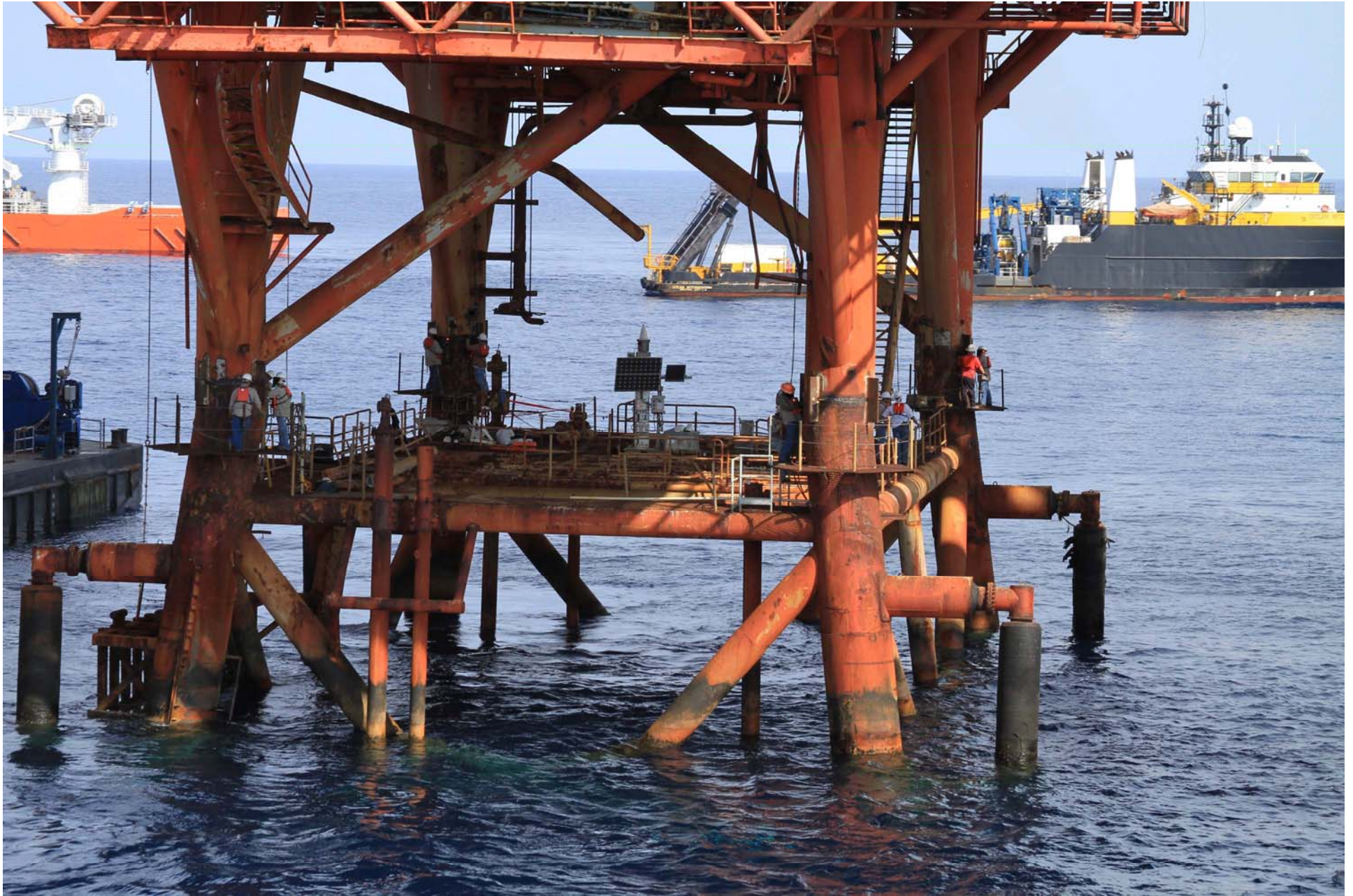
By 10:00, the welders are at work making their final cuts on the legs.
