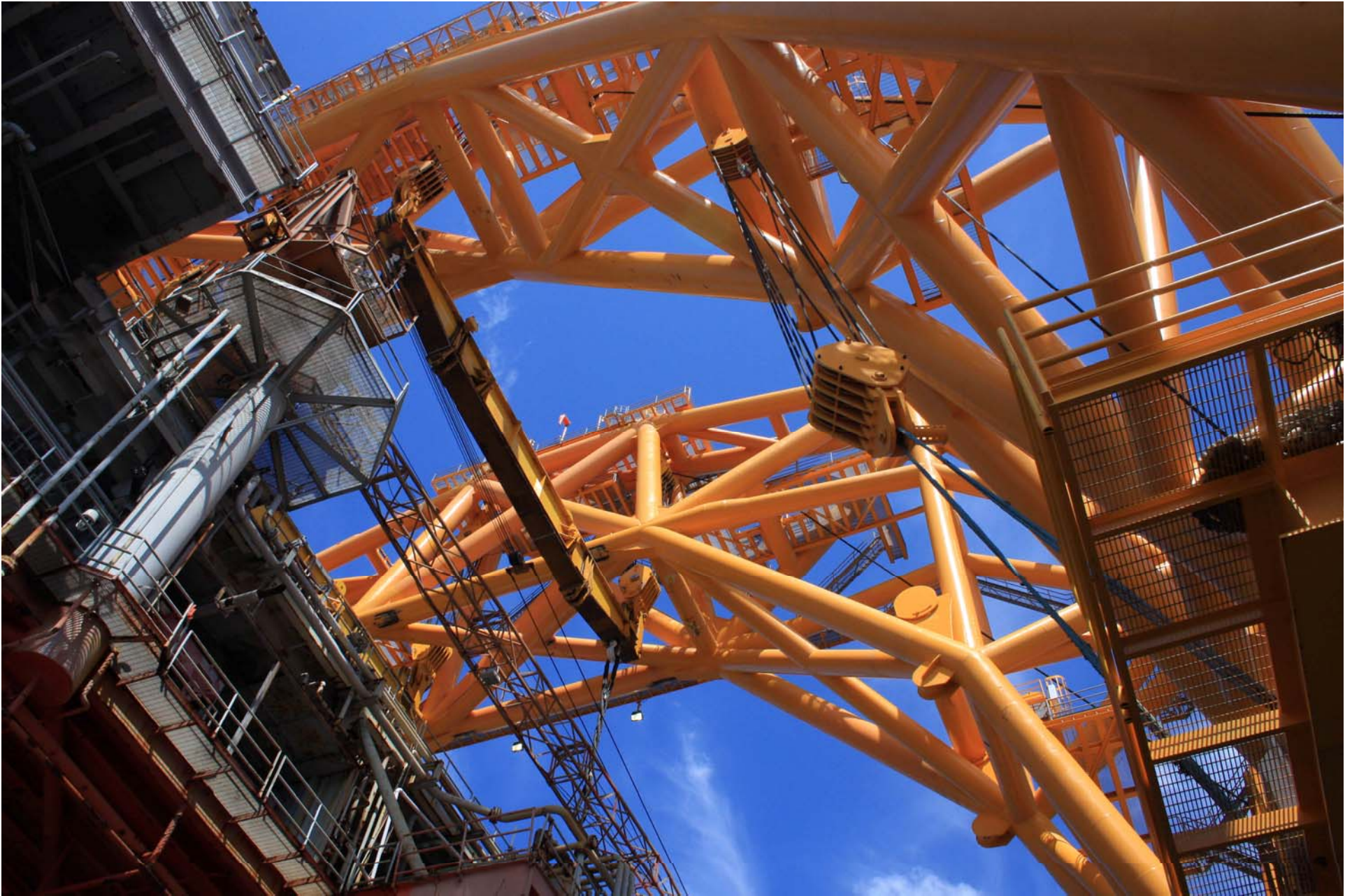
3:15 PM. The slings are unhooked from the topside. This view from the deck of the VB 10000 shows ample clearance, even for the large topside.
